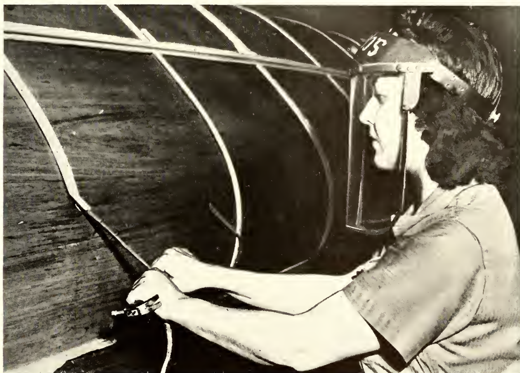
FIGURE 5-57.—Cotton webbing under nailing strips facilitates removal of the strips and nails.
